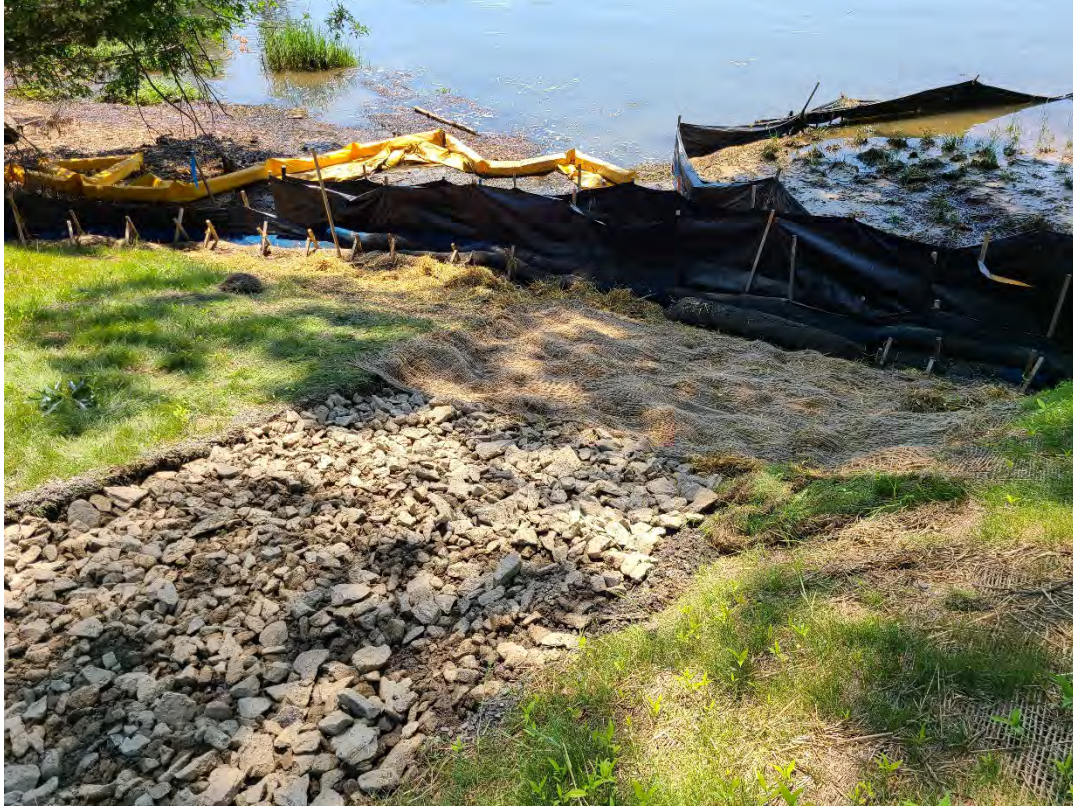
Fig 17: Corrective action repairs to gravel path below man hole at Gundalow landing/east side of the Bay. Viewing southwest. (07-01-20).
