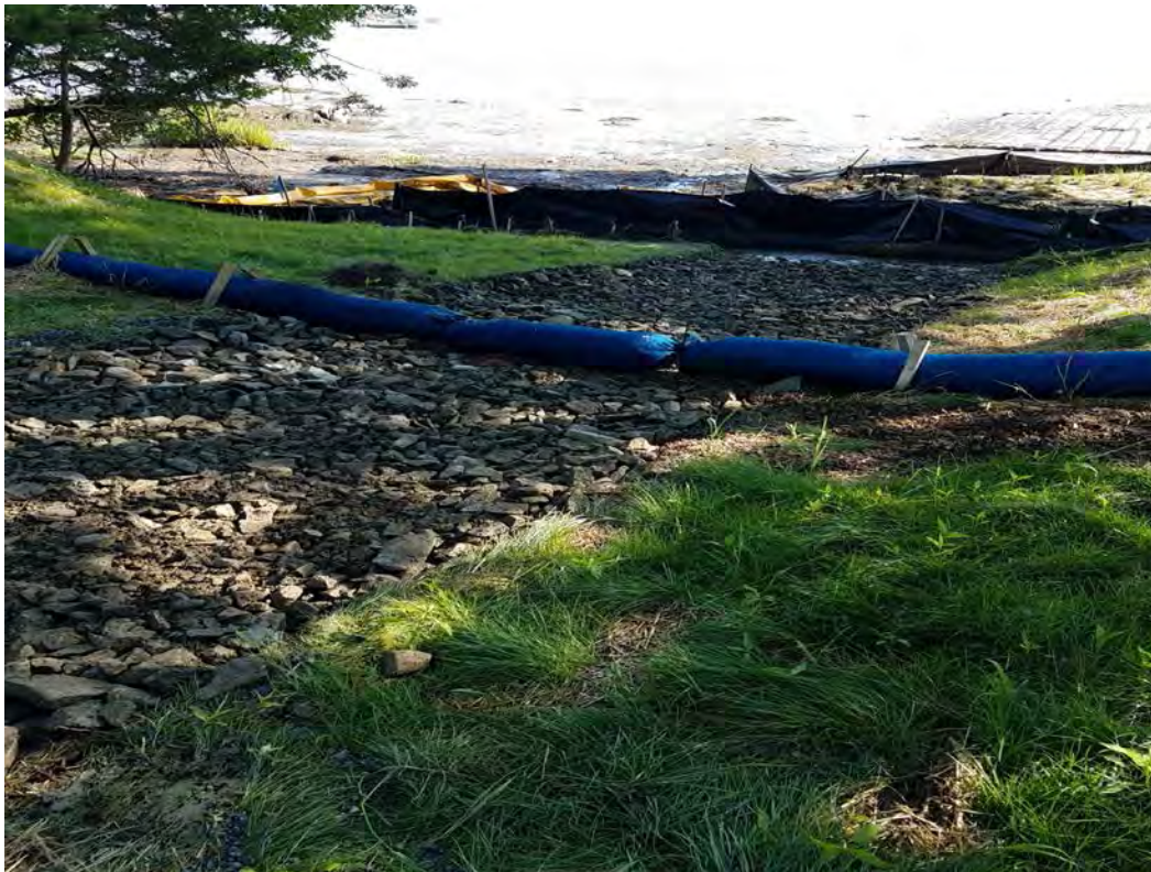
Fig 18: Corrective action repairs to gravel path below man hole at Gundalow landing/east side of the Bay. Viewing southwest. (07-01-20).
