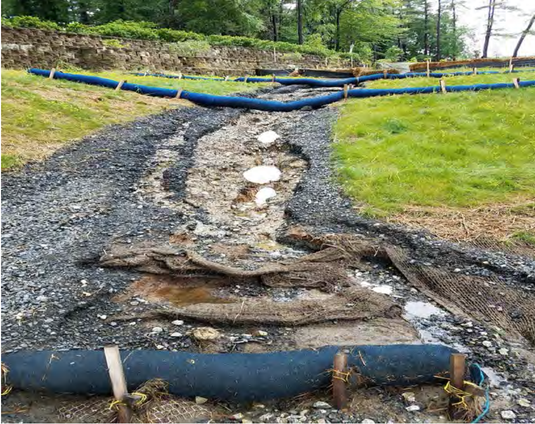
Fig 13: Gravel path at Gundalow landing/east side of the Bay washed out due to the rain event on 06-30-20. Viewing east. (07-01-20).
