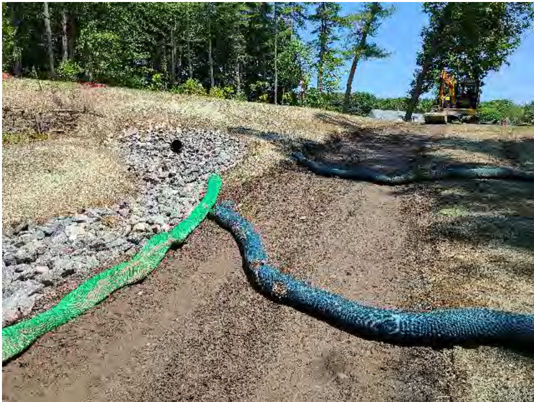
Fig 20: Repairing gravel path/culvert swale above man hole at Gundalow landing/east side of the Bay. Viewing east. (07-01-20).
