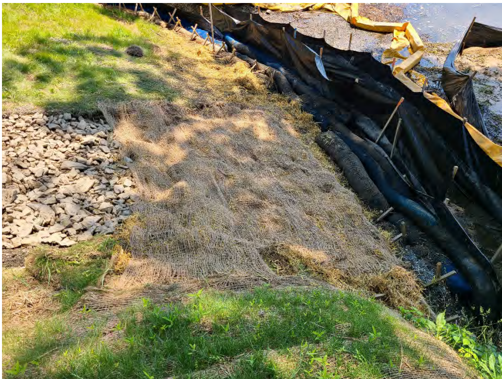
Fig 16: Corrective action repairs at toe-of-slope/intertidal zone at Gundalow landing/east side of the Bay. Viewing southwest. (07-01-20).
