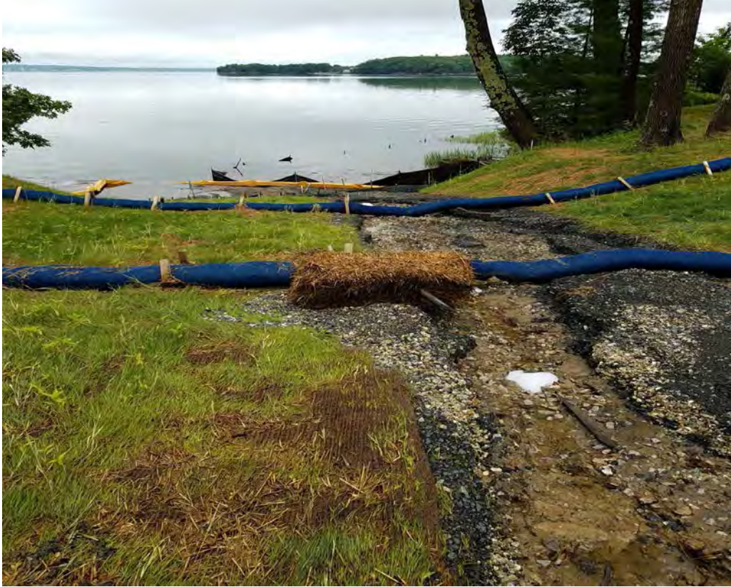
Fig 15: Gravel path erosion and deposition into the intertidal zone at Gundalow landing/east side of the Bay. Viewing west. (07-01-20).
