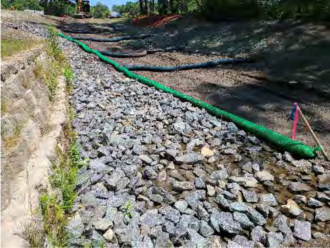
Fig 19: Rye Beach Landscaping repairing gravel path above man hole at Gundalow landing/east side of the Bay. Viewing east. (07-01-20).
